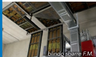
blindo sbarre F.M.
